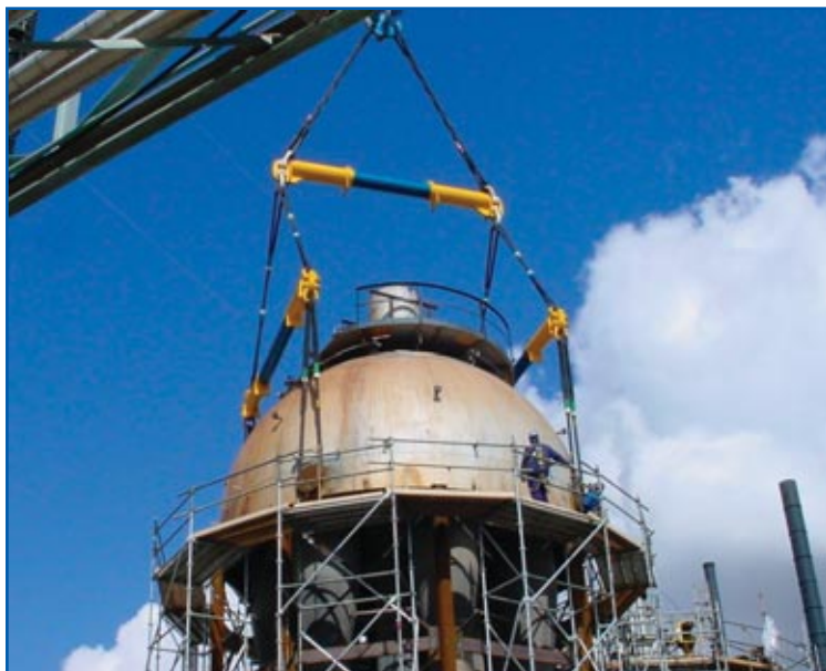
Lifting a regenerator head into place at ExxonMobil refinery in Billings, Montana
