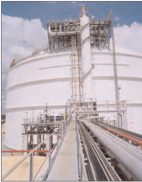
Figure 3: The storage tank and send-out system
