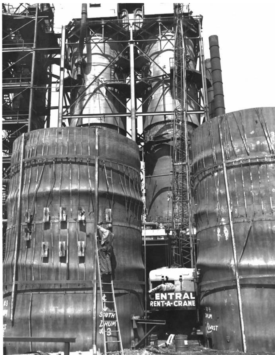
Fig. 2 — Extreme example of a coke drum shell bulging. Originally built in 1954, it was replaced in 1961.
