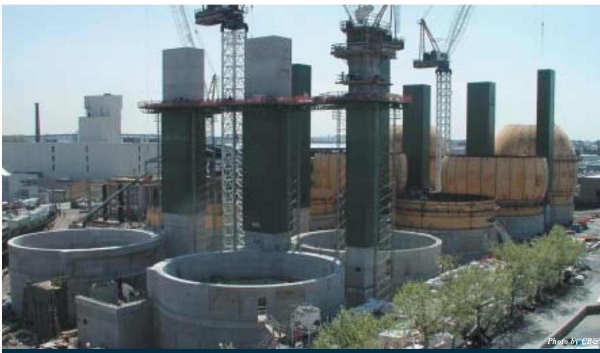
Figure 3. The Newtown Creek wastewater treatment plant includes eight egg-shaped digester vessels and two storage tanks.
