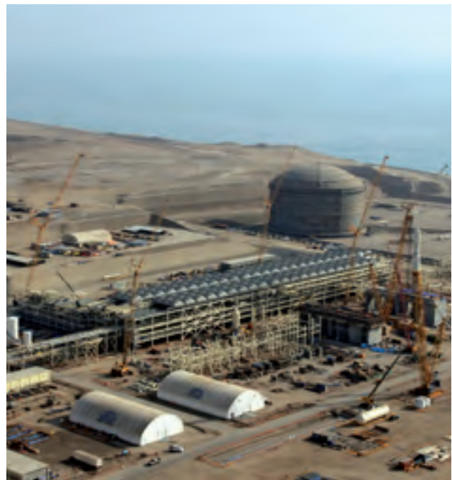
CB&I and Peru LNG have formed a joint team to start-up and initially operate the 4.5m t/y plant, which is under construction at Pampa Melchorita
