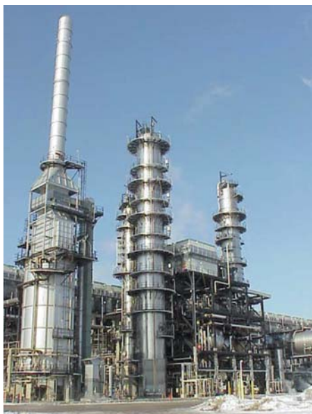
Irving Oil CDHydro/CDHDS unit located at St. John, New Brunswick, Canada
