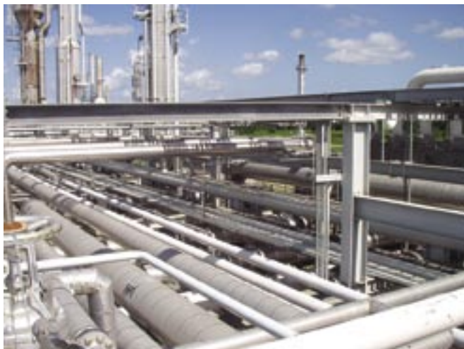
FIG. 2 The upgrade to the gas plant in the Caribbean included 230 piping tie-ins.
